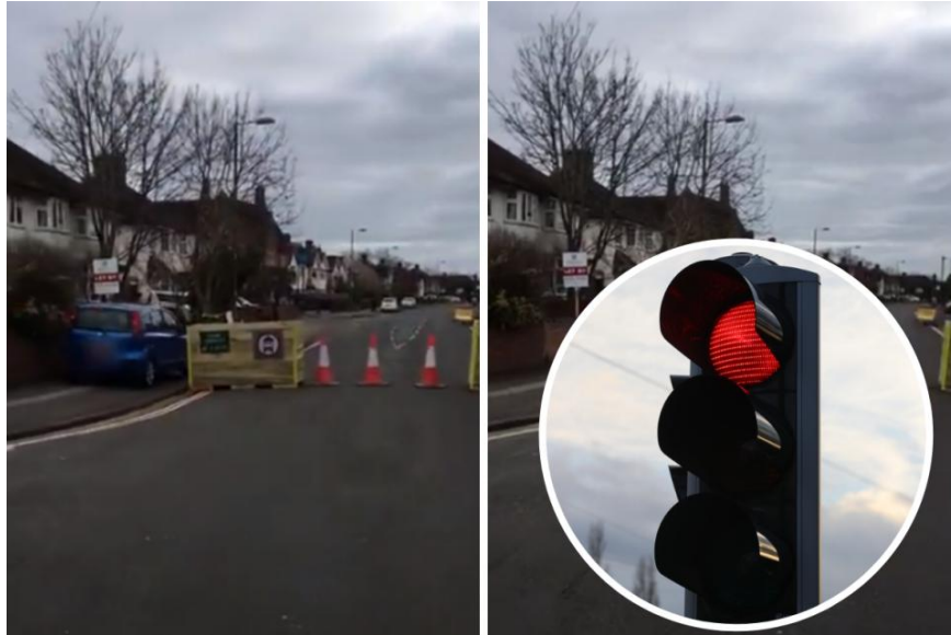
Figure 3: Frustrated motorist drives onto pavement to get around barrier
